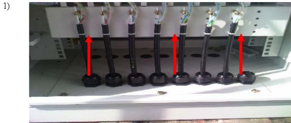
E-Side Cable coming from the bottom (plinth)
