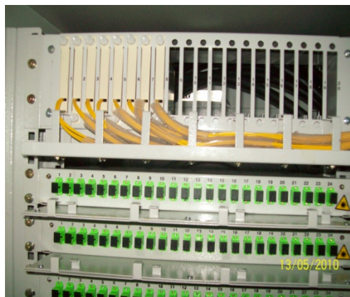
8. Proper arrangement of cables using spiral
