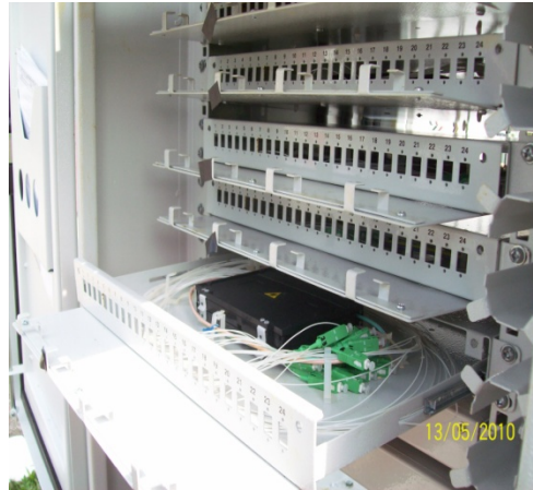
2. SC 24 core panel before installing adapters and splitters
