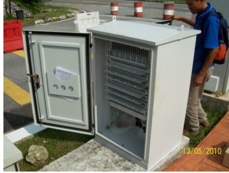
2. FDC before installing adapters and splitters
